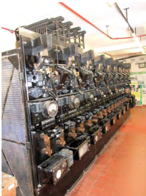
The Ipswich switchgear panel which still survives after nearly 90 years! Also see the close-up on page 14. [Stephen Cobb]
